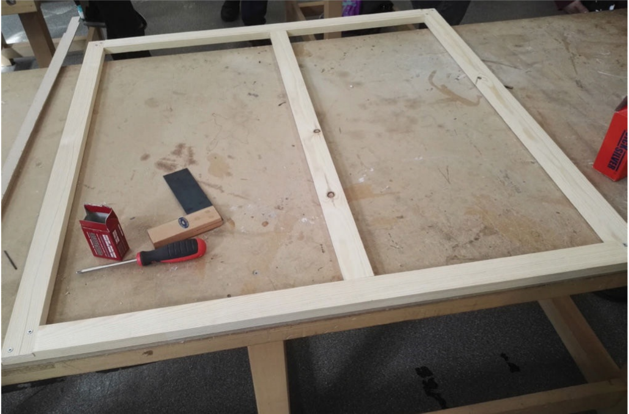
Care is taken to measure the diagonals to ensure that the strainer is square.
