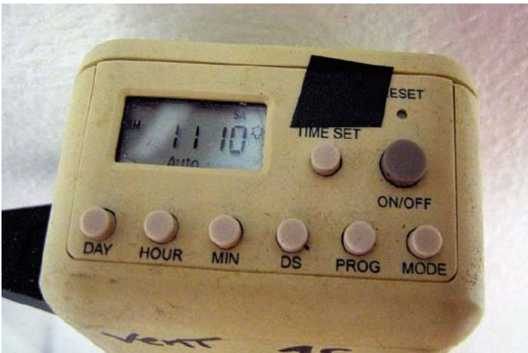
Always cover any power lights or LEDs on any electrical equipment in your
