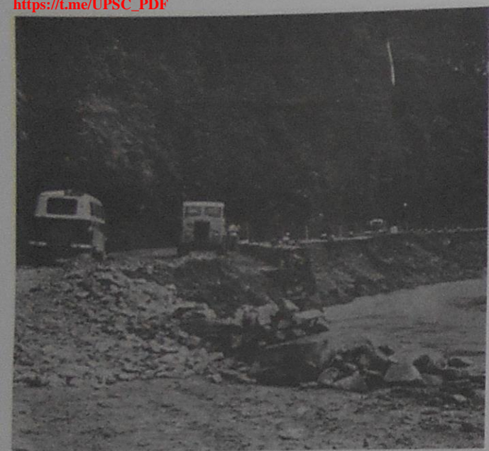
4.C A landslide after flood has damaged the road Jabatan Penerangan Malaysia
